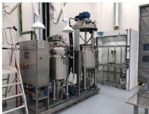
New encapsulation production line installed by Carinsa
